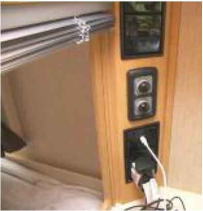
Heater controls were placed by the side dresser and also a second TV point was placed here to. Battery/lights panel was placed just inside the doorway.
